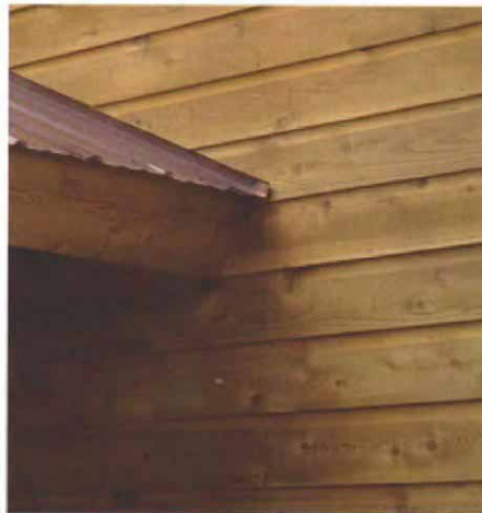
Divert runoff away from sidewalls. A gable roof that abuts a sidewall can direct water behind the siding at the junction along the roof's edge. Thwart the problem with a flap of flashing that directs runoff away from the wall.
